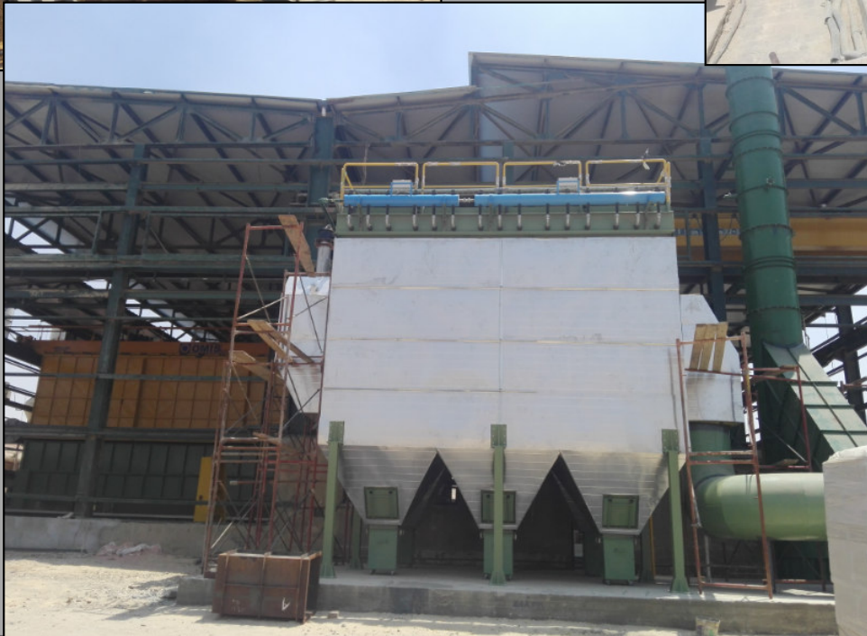
Hot Dip Galvanizing Plant
