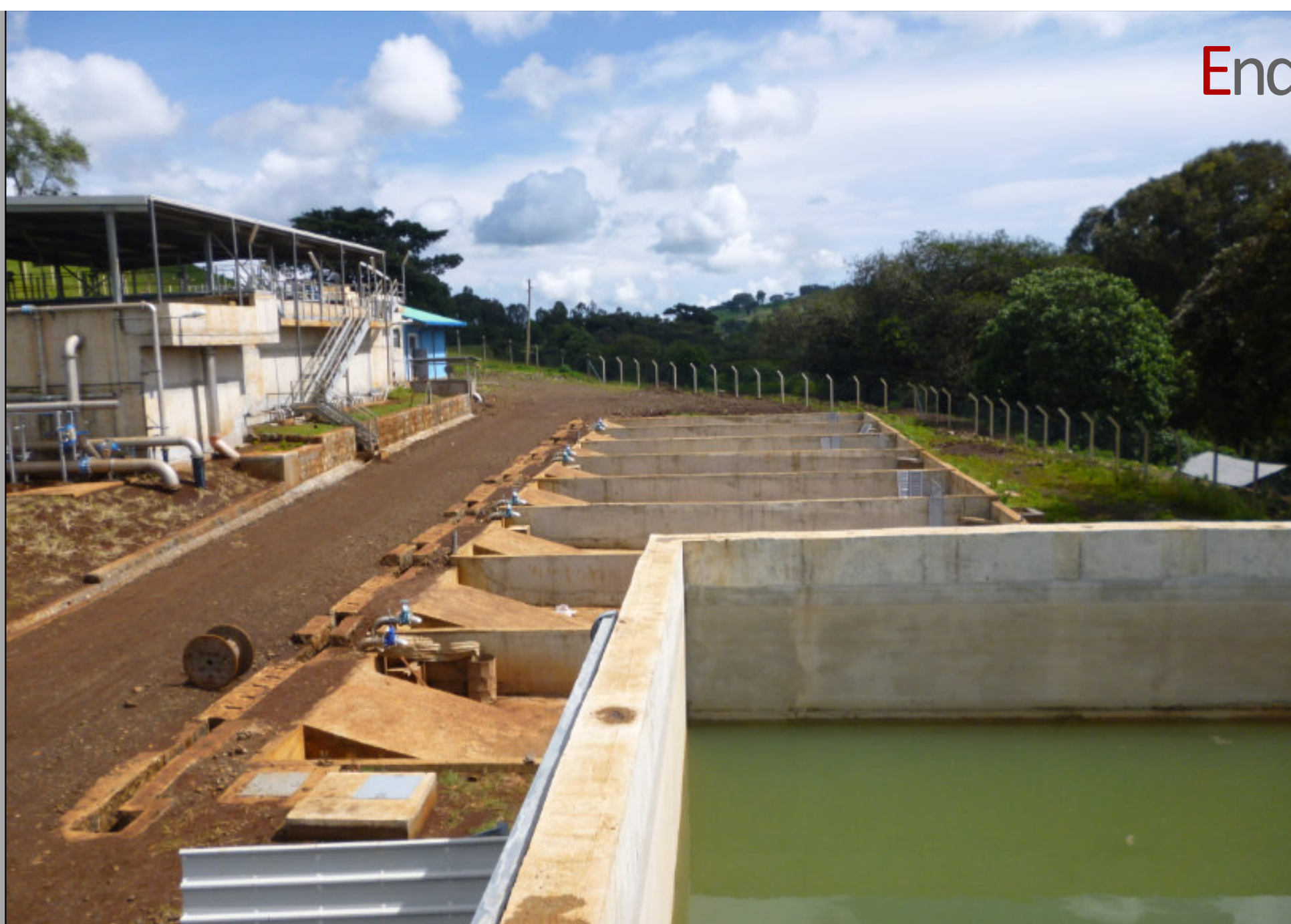
Dembidollo Water Treatment Plant Ethiopia
