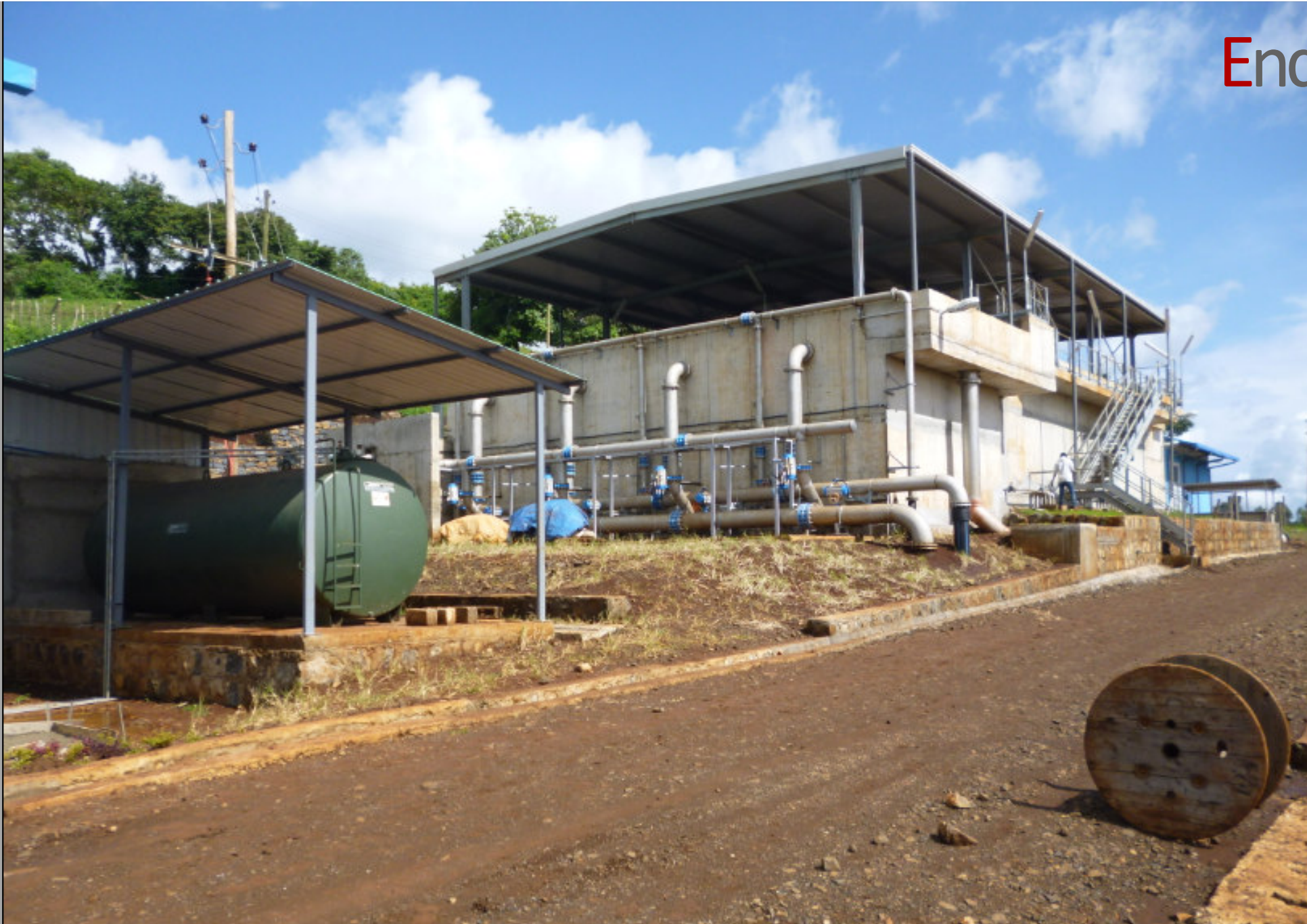
Dembidollo Water Treatment Plant Ethiopia
