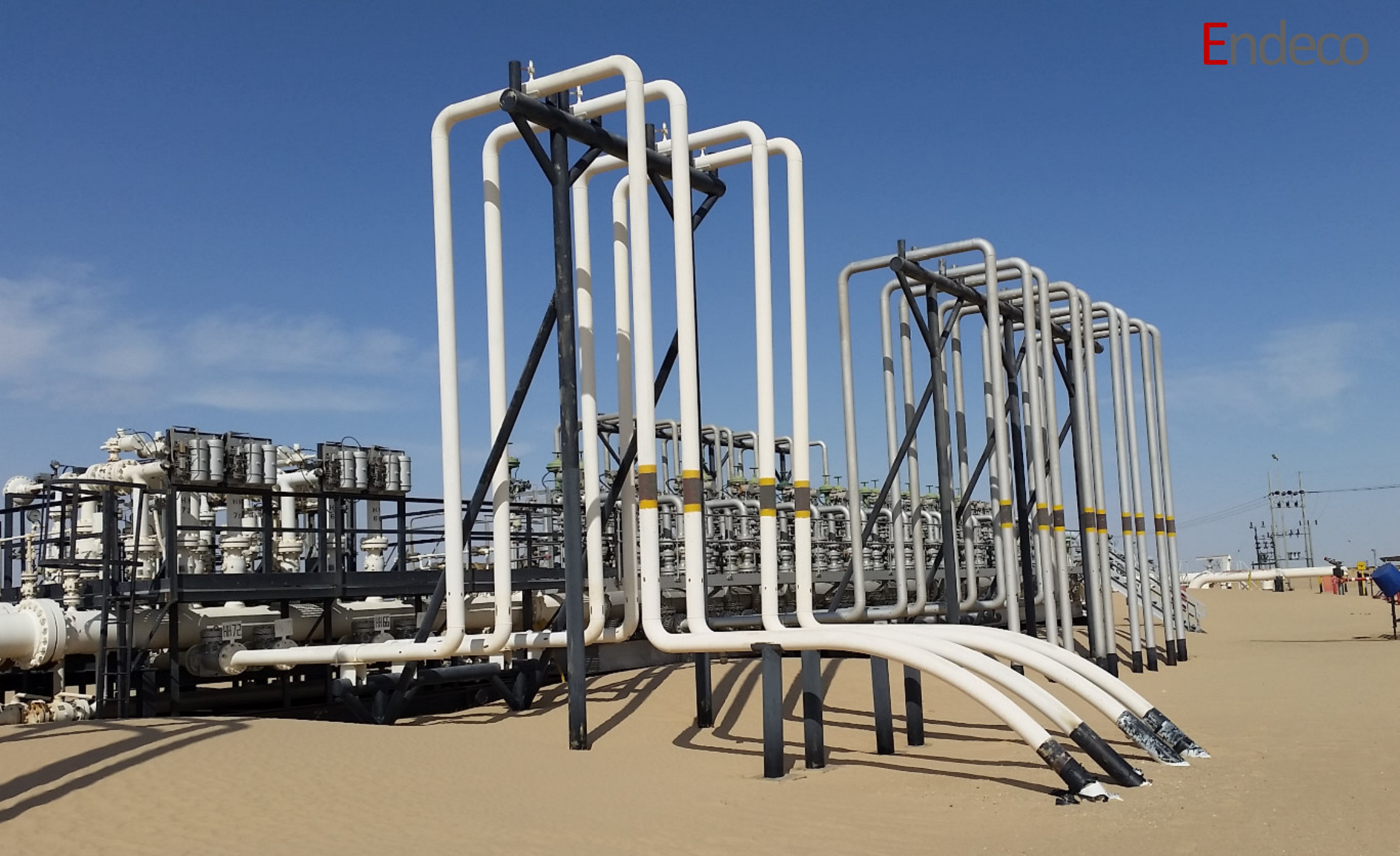
MESSLA MANIFOLDS INSTALLATION
