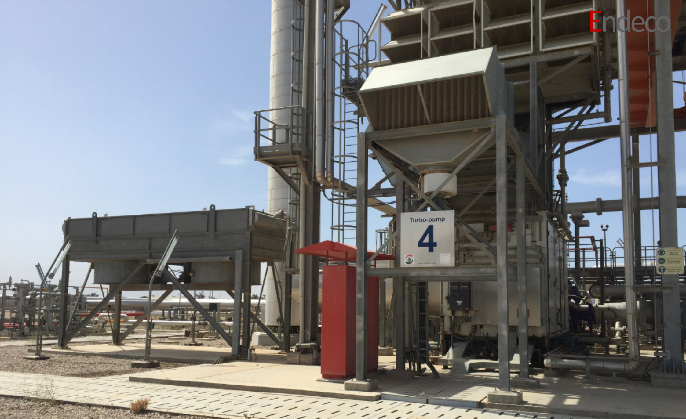
Zubair Turbogas Oil Pumping Station
