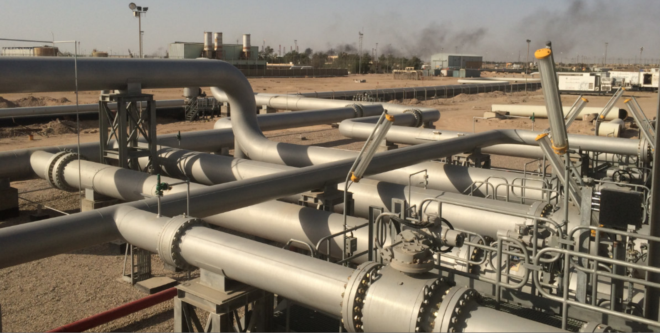
Tuba Turbogas Oil Pumping Station
