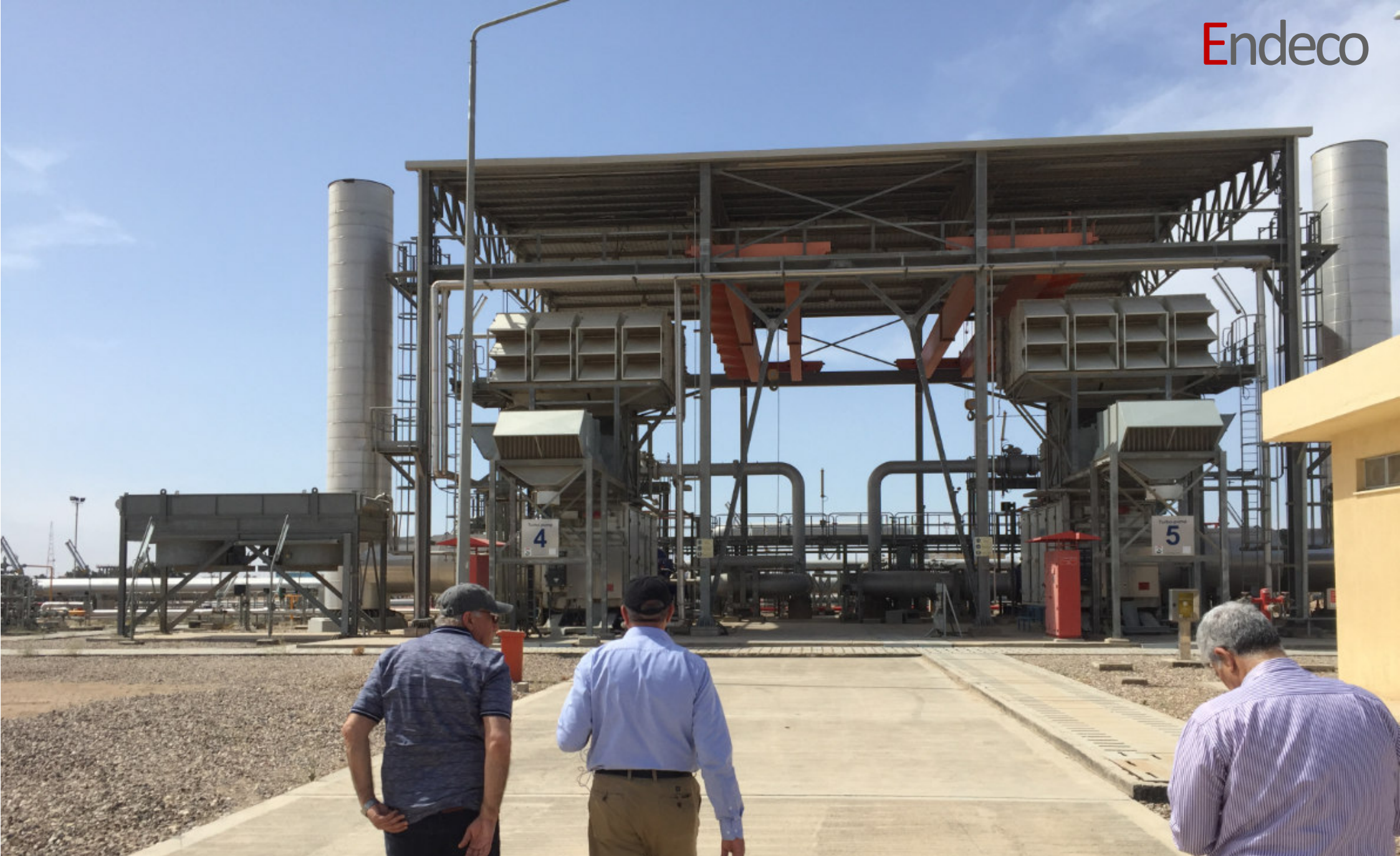
Zubair Turbogas Oil Pumping Station
