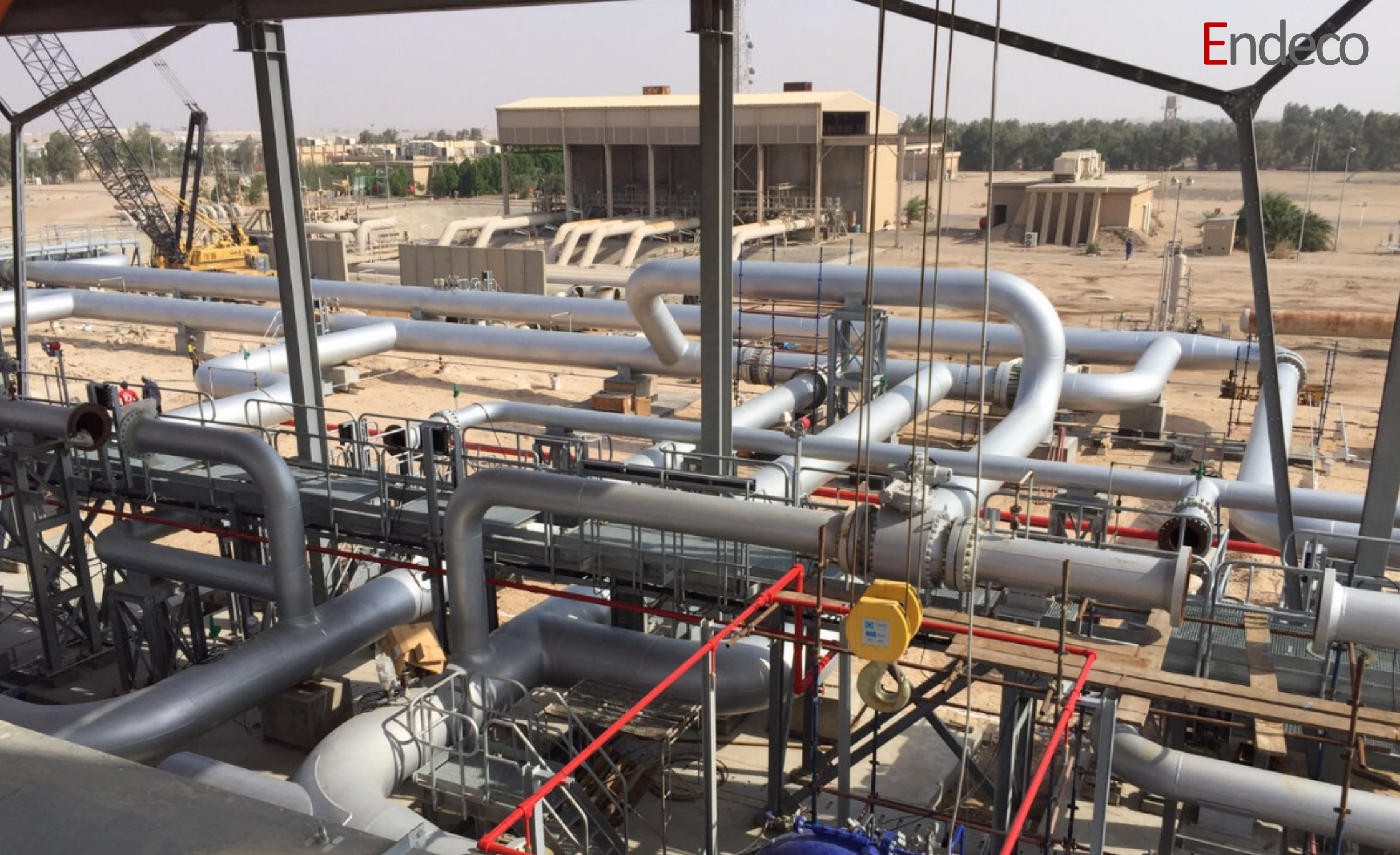
Tuba Turbogas Oil Pumping Station
