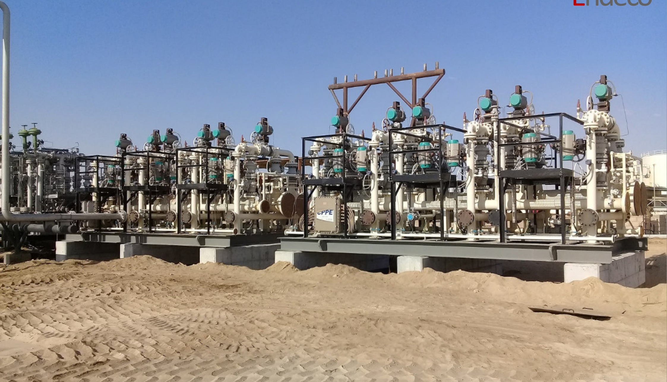
MESSLA MANIFOLDS INSTALLATION
