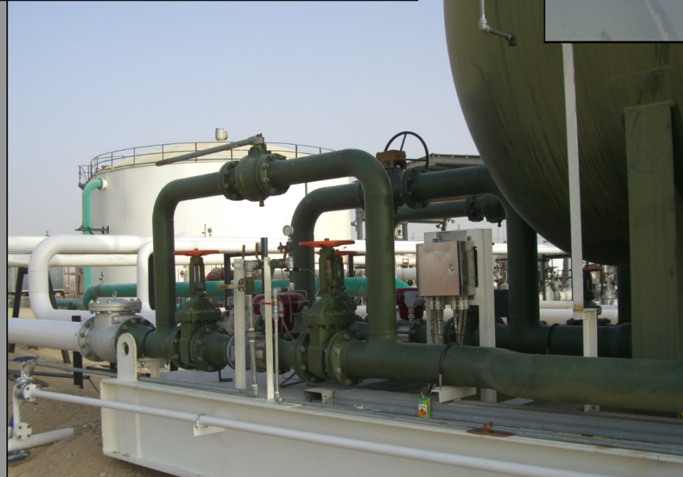
THREE PHASE SEPARATOR
