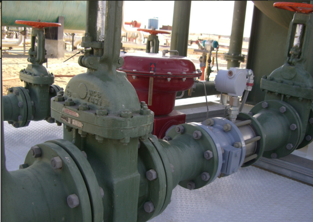
THREE PHASE SEPARATOR
