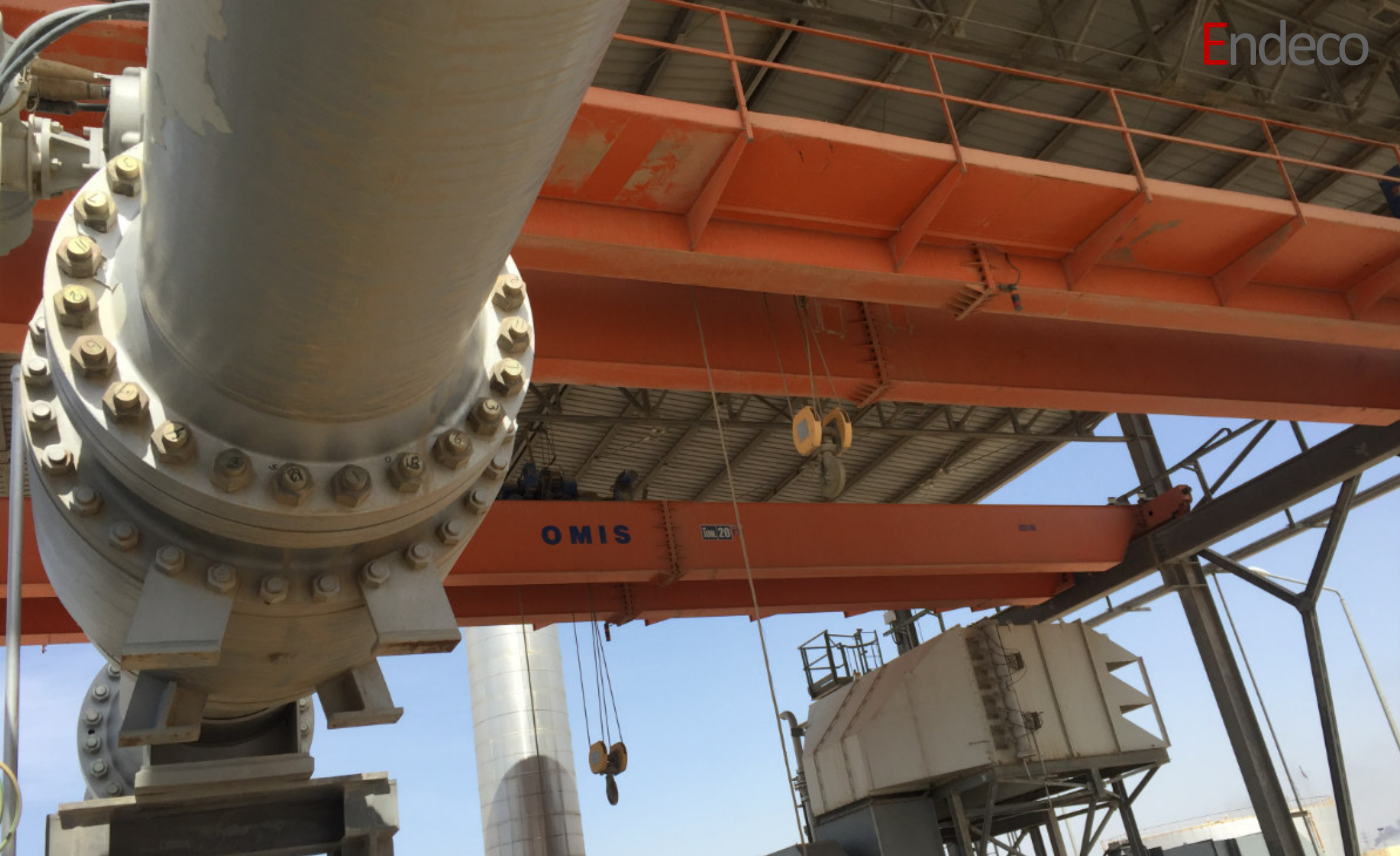
Zubair Turbogas Oil Pumping Station
