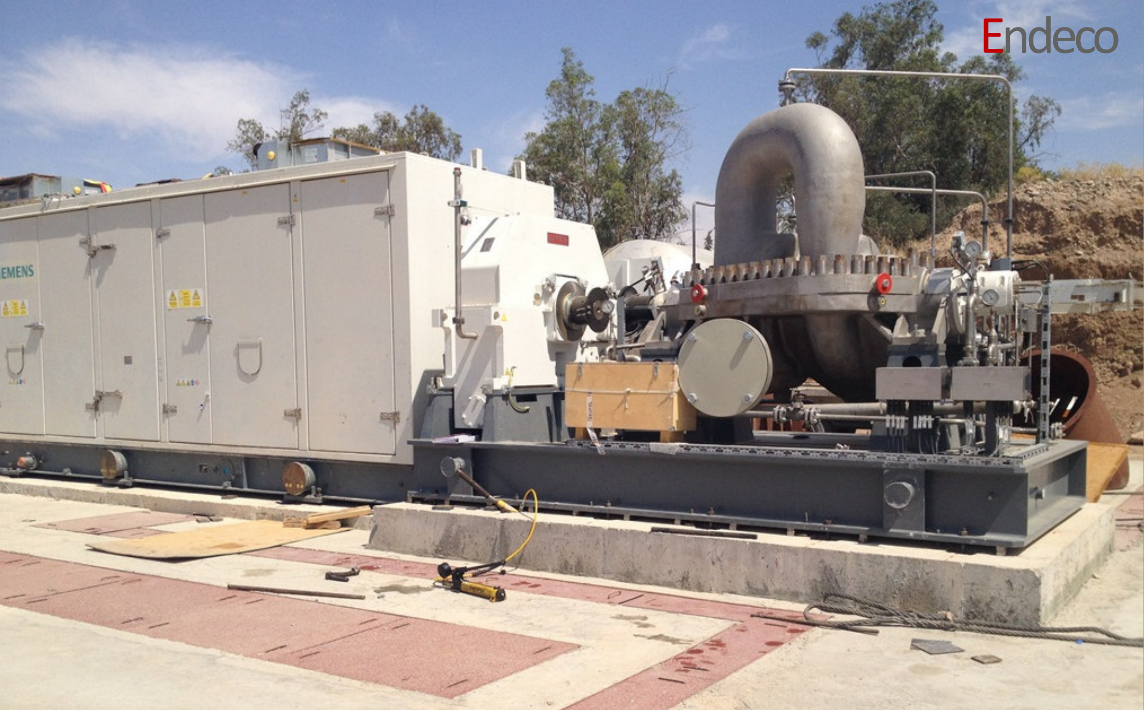
WATER INJECTION STATION
