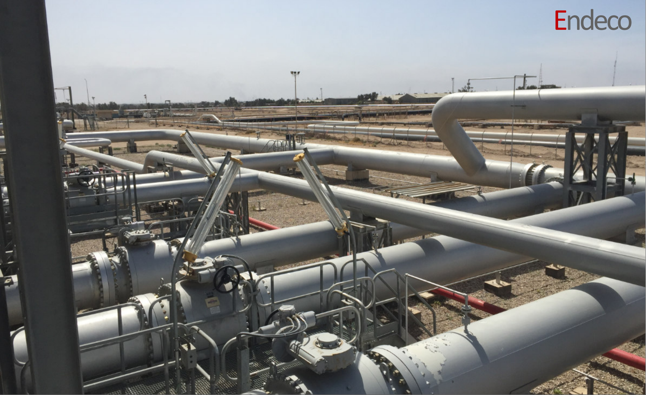
Zubair Turbogas Oil Pumping Station
