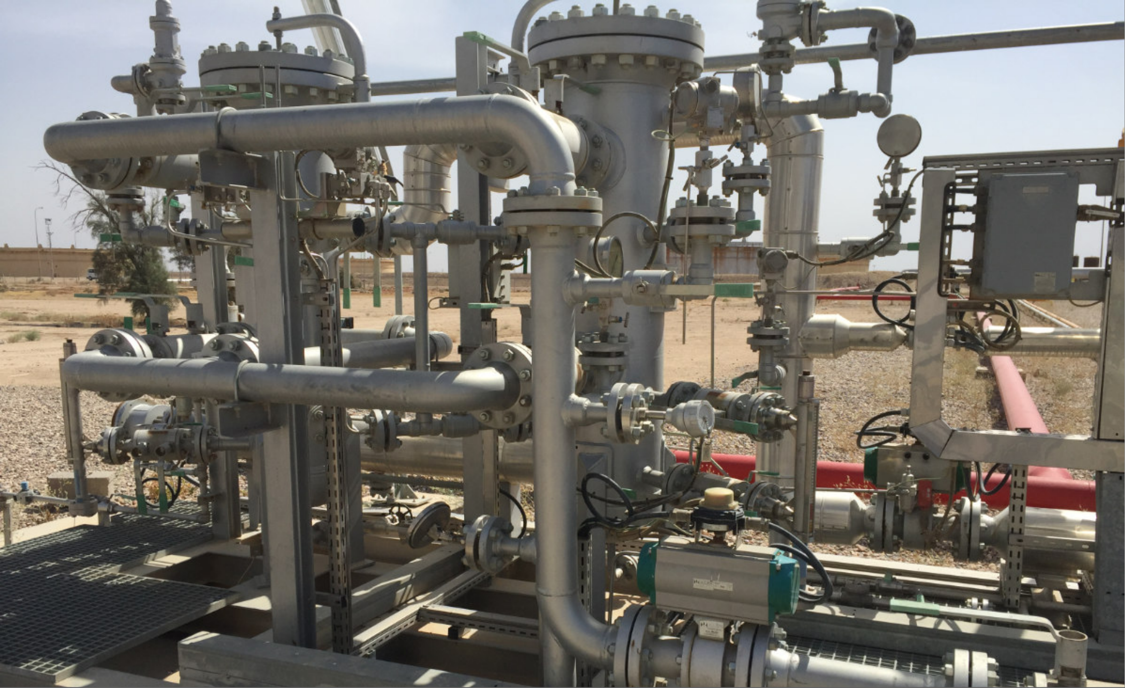
Zubair Turbogas Oil Pumping Station
