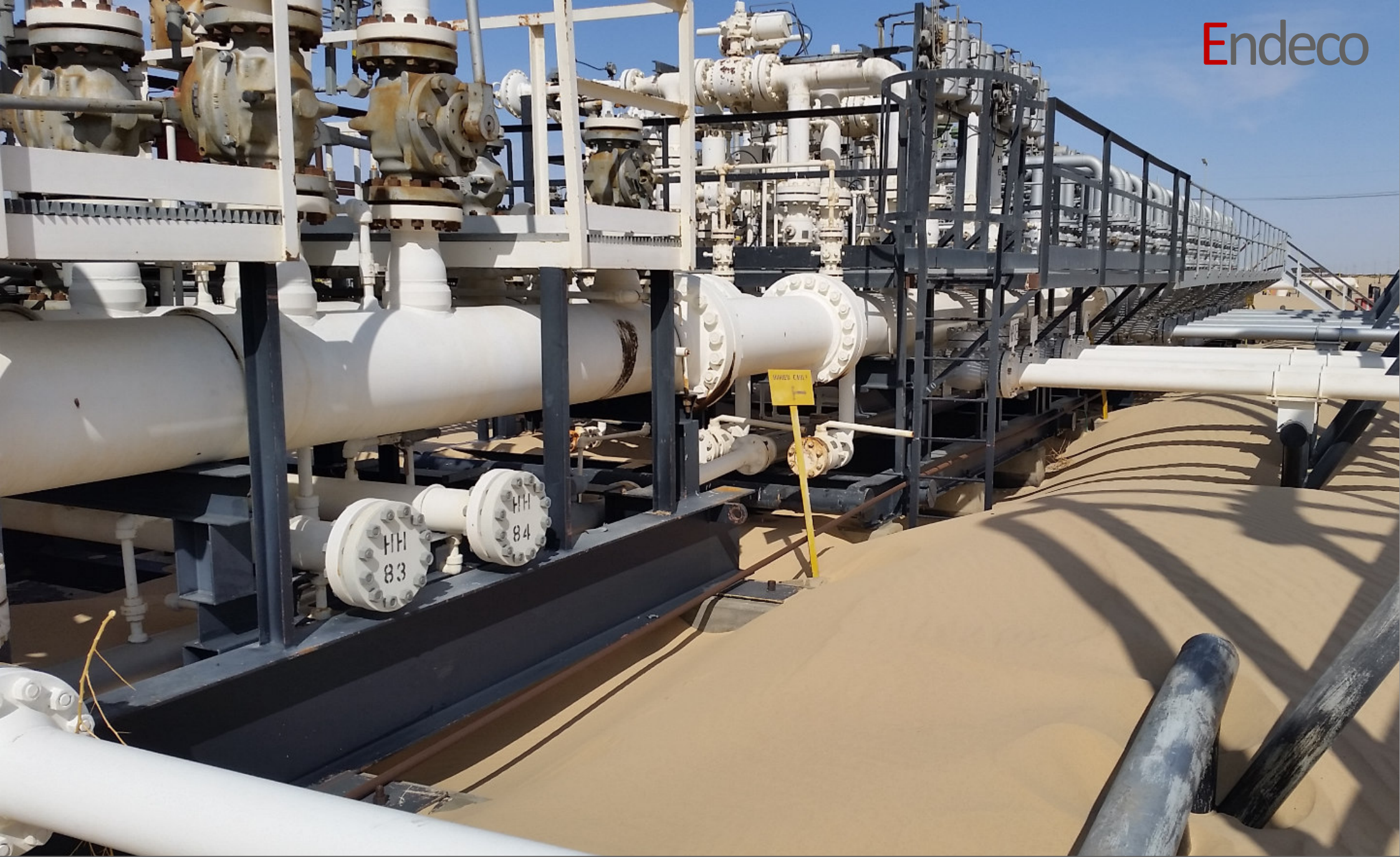
MESSLA MANIFOLDS INSTALLATION
