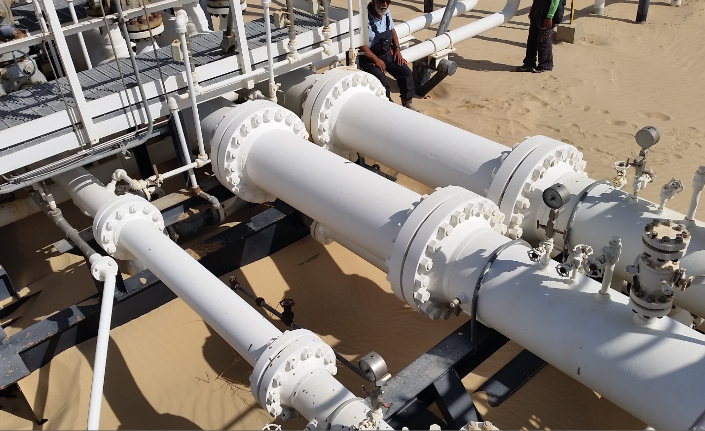
MESSLA MANIFOLDS INSTALLATION
